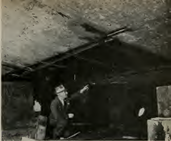
David C. Buchan, boss shipwright, checking to see that there are sufficient shores under the President Taft while damaged sections of shell plates and floors are being removed.
